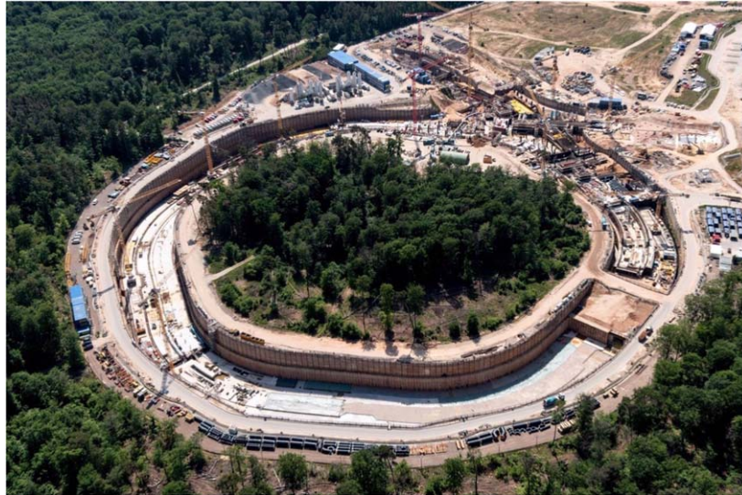
Figure 4. The FAIR construction site in spring 2020. The picture shows the progress in civil construction for the SIS 100 tunnel, the ‘transfer building’, where the beam delivery from the existing and upgraded GSI accelerator chain into the SIS 100 and also the delivery from the SIS 100 to the various FAIR experimental sites will occur, and the cave which will hold the CBM experiment. Now, in winter 2022/3 the SIS100 tunnel is closed and the civil construction on the south campus (upper right part in the figure) has nearly been completed. The first science experiments are scheduled to start in 2027. Credit: GSI.
