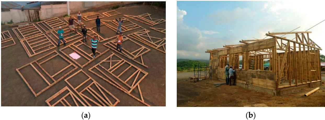
Figure 10. Prefabricated panels; bamboo house under construction. (a) Frame ready for assembly. Source: INBAR; (b) Assembly on the site. Source: Bambuksa [bambuksa.org].
