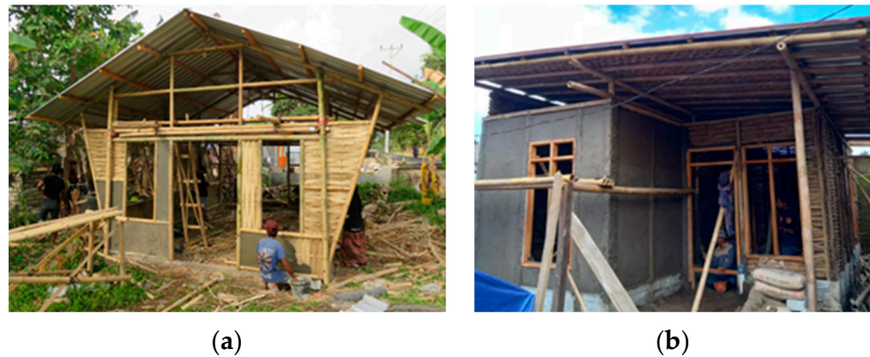
Figure 6. Example homes in Indonesia. (a) Bamboo house with two floors in Lombok. Source: ITB and UMRAM [28]. (b) Bamboo house with gypsum plaster in Cianjur, West-Java. Source: ITB [28].
