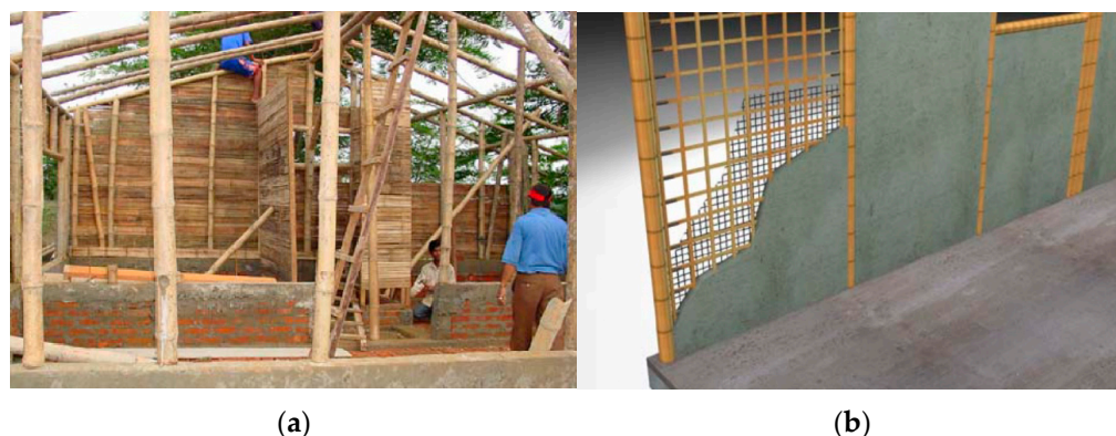
Figure 2. (a,b) Frames for house construction. (a) Wall with infill frames. (b) Sources: INBAR.
