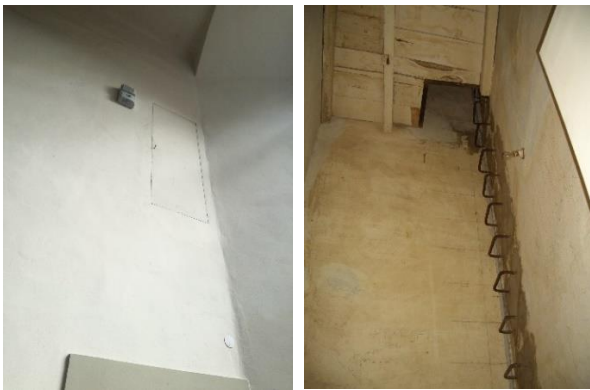
Figure 6. Figure 7. The odd access to the hidden space in the southern façade.
