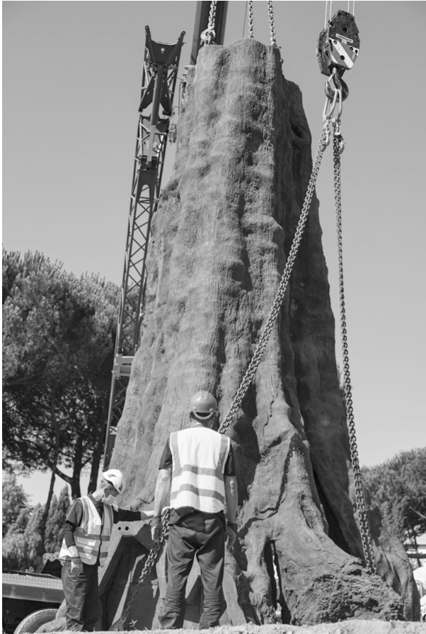
Figure 2: Installation of Ai Weiwei's Pequi Tree (2018–20; cast iron; 32.4 x 11.5 x 9.8 m) at the Serralves Museum of Contemporary Art, Porto, for the exhibit Entrelaçar/Intertwine (July 23, 2021, to July 9, 2022). Image courtesy of Serralves Museum of Contemporary Art and Ai Weiwei Studio.
