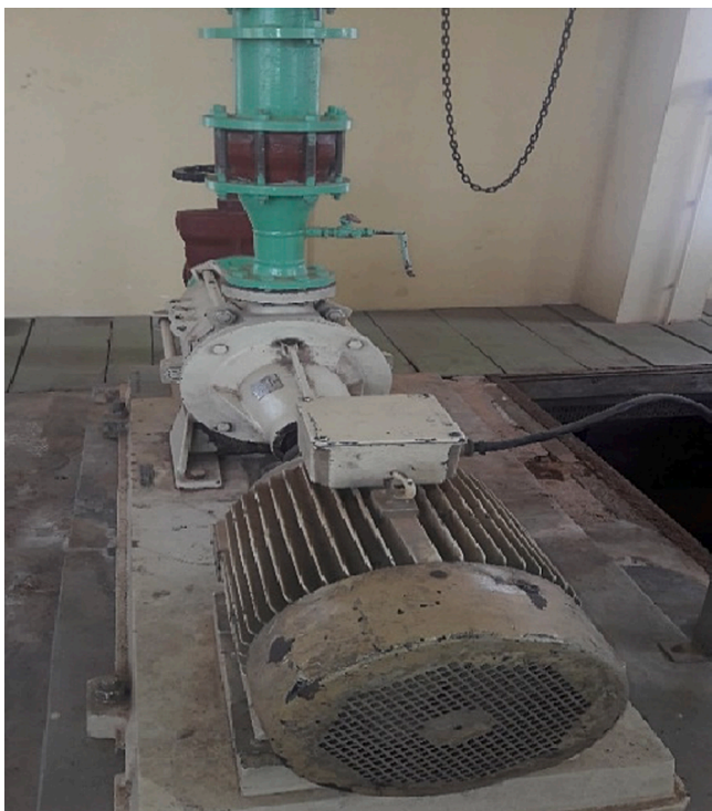
Fig. 2. An abandoned booster pump in Accra.
