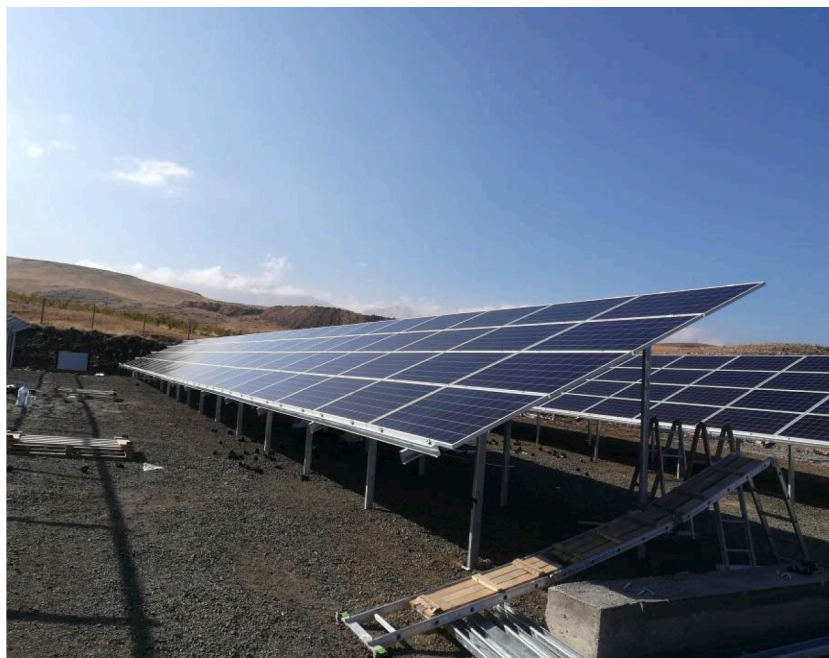
Fig. 1. 500 kWp grid-connected solar power plant at Iğdir University.
