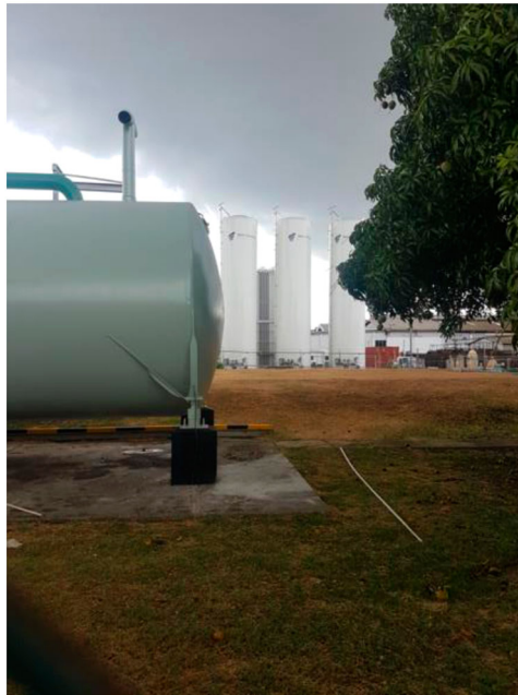
Figure 3. Part of the Red Stripe energy system (LNG). Source: Pilo' (2019).
