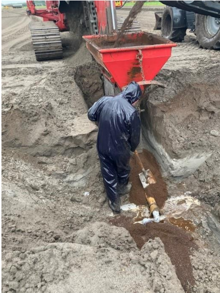
Figure 6-1 ICS filter construction around drains in a flower growing farm in the west of the Netherlands
