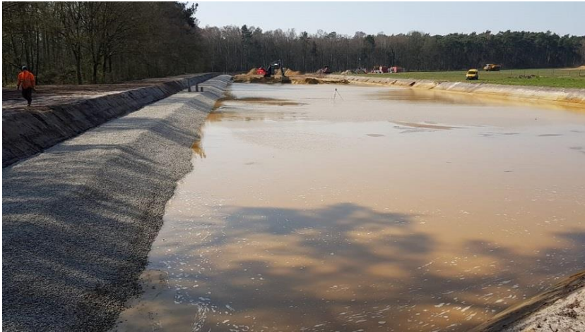
Figure 6-3 ICS filter and basin, three drains are covered by ICS which filters the water
