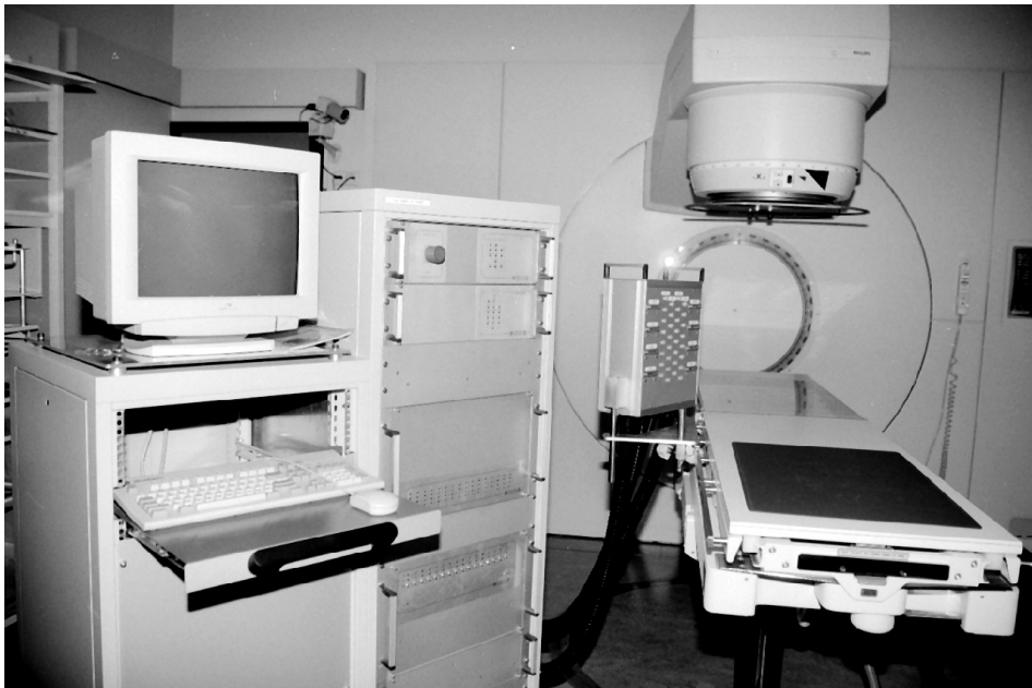
Figure 2.2: Photograph of the assembled IHT machine. The following subsystems are shown: to the left, the system console. In the cabinet next to the console, the power generator, switchboards and dedicated controller. During treatment, the detached connection box is located near the patient.
