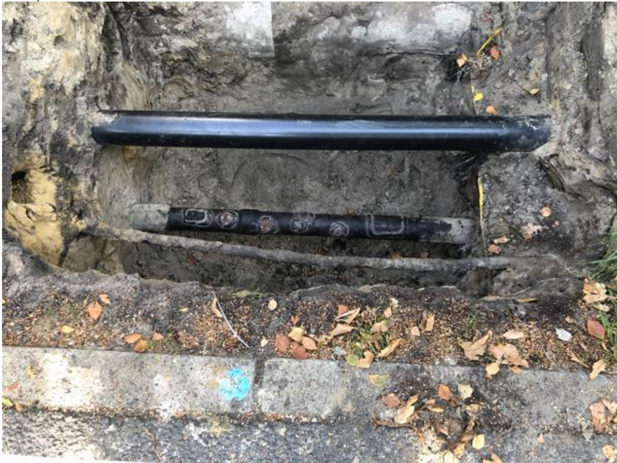
Figure 4.S9. The LDC reported 6 leaks on the pipeline at this location with total leak area of 5 cm 2 , HH013.
