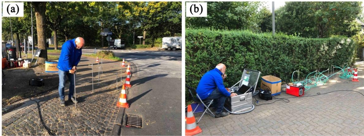
Figure 4.S7. Inserting suction probes into holes drilled above the pipeline at location HH009 (a), and quantification in action at location HH002 (b).
