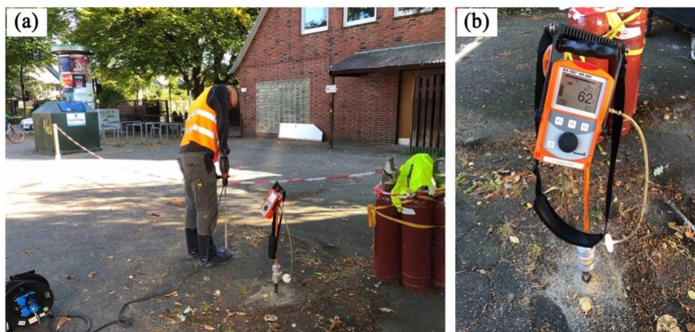
Figure 4.S3. Drilling holes around the surface-projected track of gas pipeline (a) and measuring the CH 4 mole percentage (b) to find the gas leak location, HH008.
