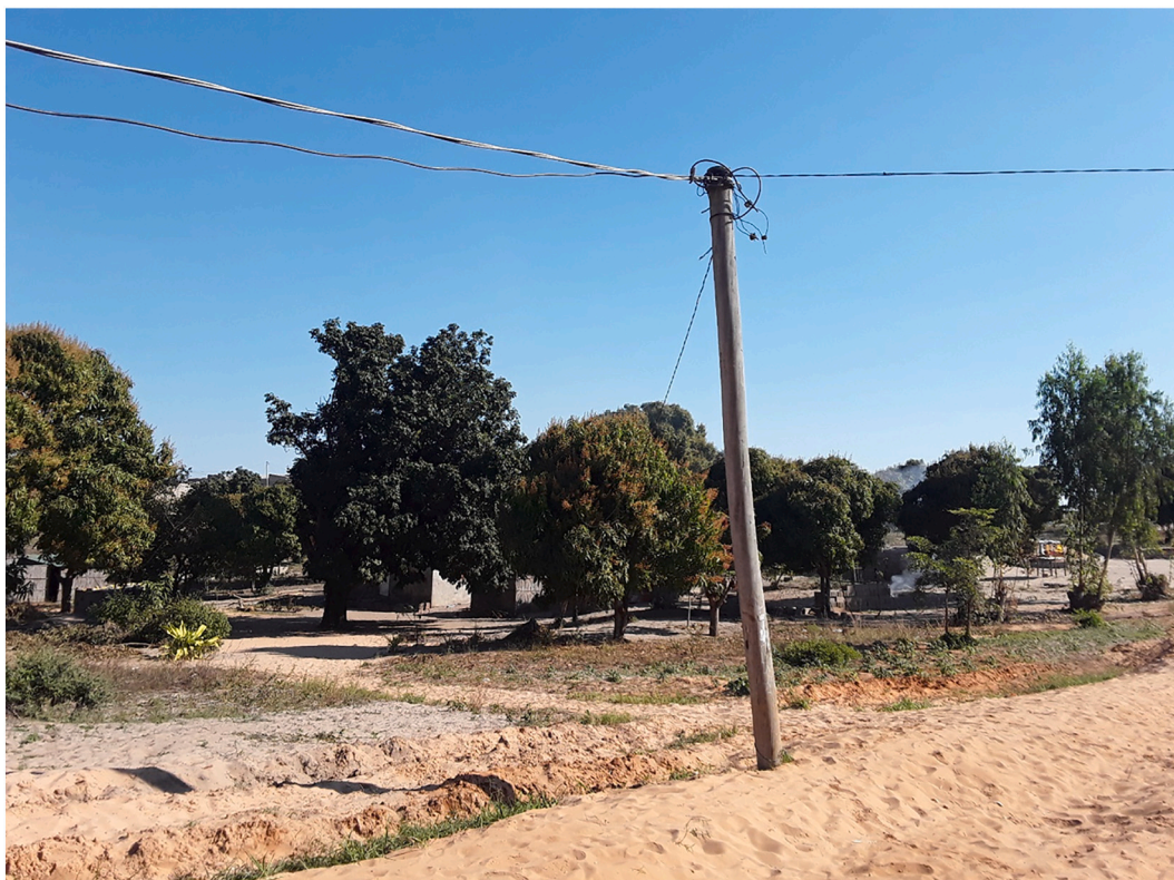
Photo 1. An example of a pole bought and installed by residents. Residents installed the pole because an initial electrification project did not cover their houses.
