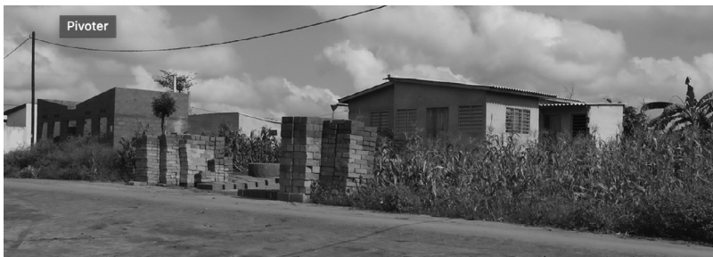
FIGURE 3.2 “Djagblé City” under construction in 2016, five years after the resettlement. Source: Photo taken by Authors, 2016.
