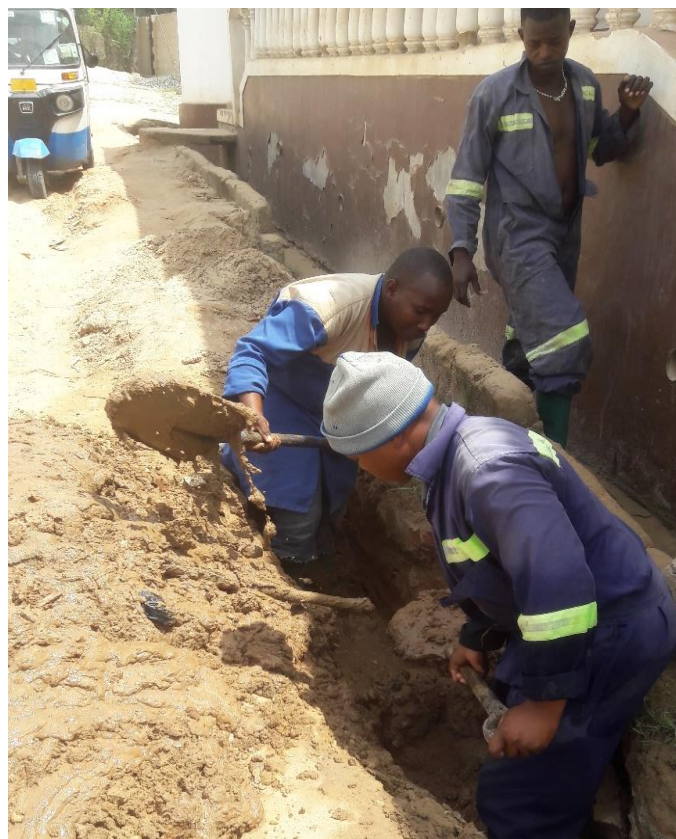
Figure 4. Pipelines under frontage of a building in Dar es Salaam.
