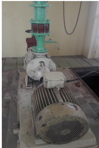
Figure 5. Malfunctioning booster pumps at Dodowa, Accra.
