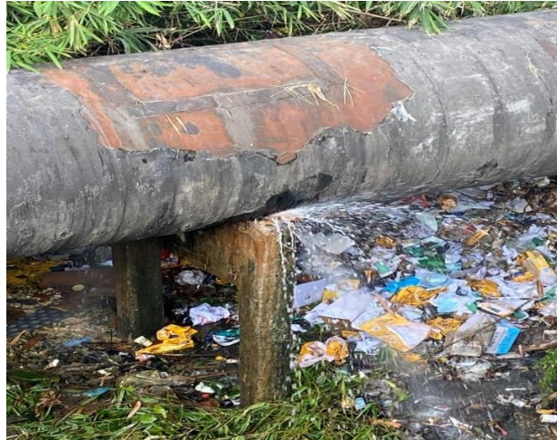
Figure 6. Leaking pipe in Dar es Salaam.
