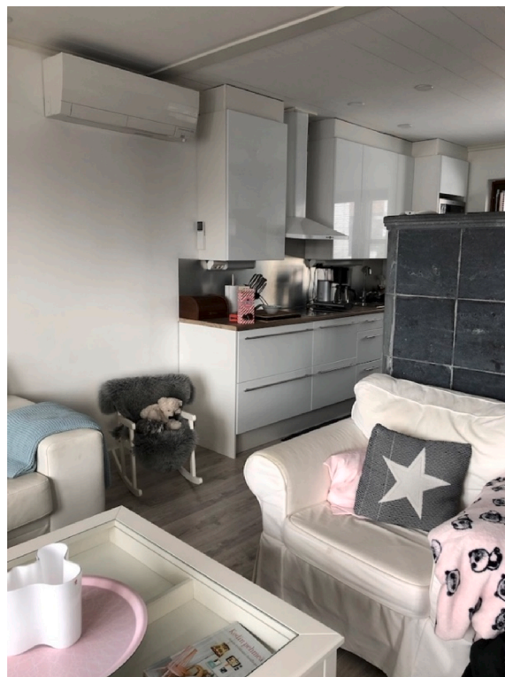
Fig. 5. An ASHP inside unit at a family home in Finland. Source: Authors.
