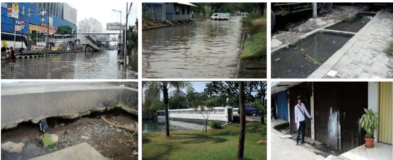
Fig. 9. The impact of land subsidence in Jakarta, e.g., tidal inundation “rob”, crack on infrastructure, the “sinking” bridge, problem in drainage, and problem of low level on the house to the road.
