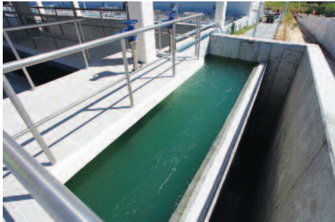
Image 5: Water aeration at the new treatment facility.
