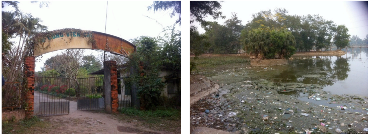
Figure 8: Degradation of infrastructure and rubbish in Cầu Đôi park (photos taken in January 2014). Photo courtesy: Tạ Thị Trâm. Source: Authors
