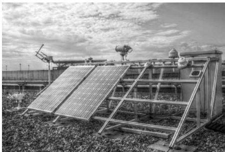
Figure 1: Experimental assembly of EKO Instruments roof-site in Den Haag, Netherlands: PV modules, radiation sensors, and instruments cabinet
