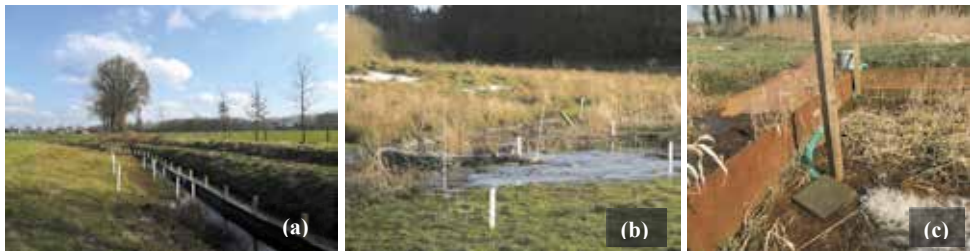
Figure 5.7. Longitudinal dam construction made of ‘Trespa’ plate material (a), a sand bag dam (b), and close-up of pump installation at the boundary of the flooding section (c).
