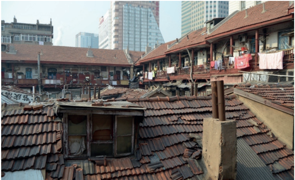
Figure 5.8 Poor living conditions in Liyuan
