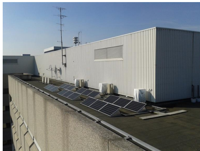
Figure 2. The experimental facility of SEAC.
