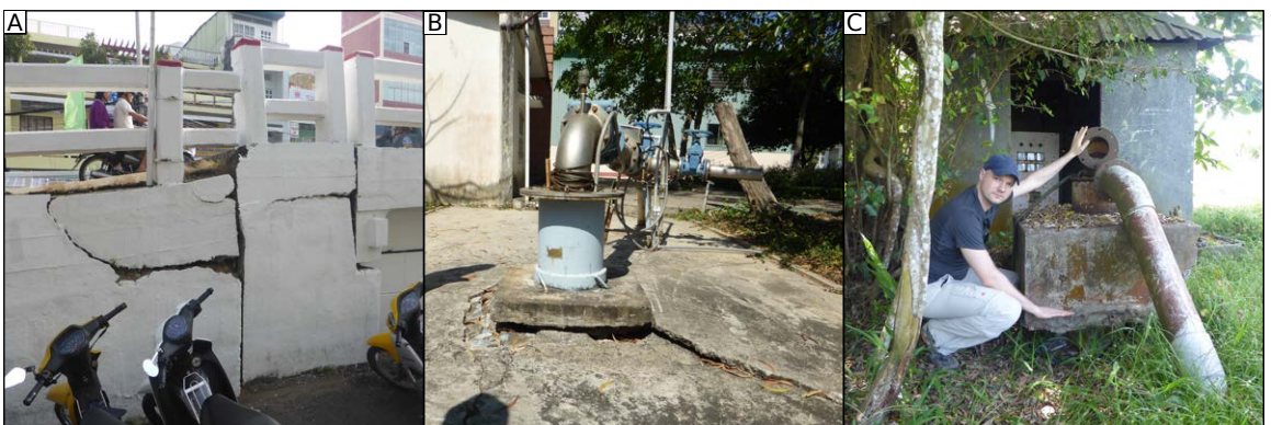
Fig. 1.7 | Evidence of subsidence in the Mekong delta. A) Cracks in a bridge ramp caused by shallow subsidence. B) Protruding groundwater well evident by the cracked concrete floor and bended pipe. C) Abandoned protruding groundwater well. The original delta surface when the well was installed is indicated by the author's right hand.
