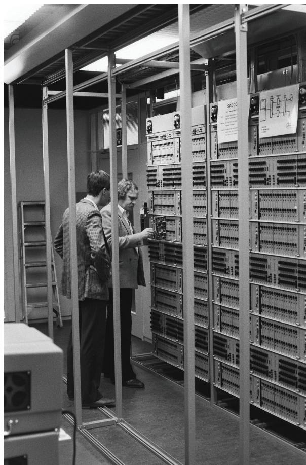
Data infrastructure at the Amsterdam location of the digital telephone exchange of PPT, the national mail and telephone service of the Netherlands (1985). Photo credit: Roland Gerrits; collection: fotocollectie Anefo, Nationaal Archief.
