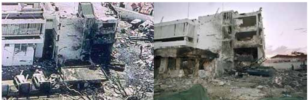
Fig 3.3 Left: the damaged US Embassy in Dar es Salaam, August 1998. 228 Right: water truck remains next to the Embassy, August 8, 1998. 229
