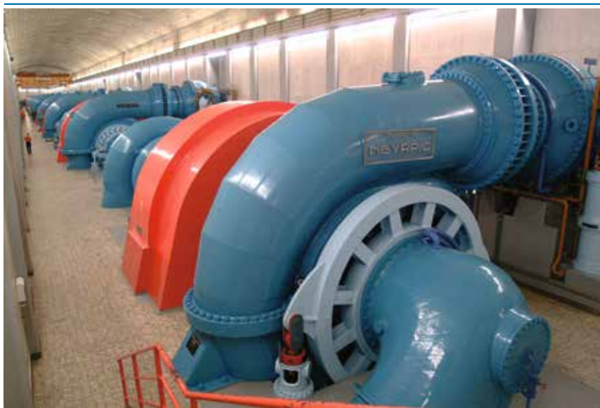
Figure 32 – PHS Vianden with horizontal rotary axes. Source: SEO (Société Electrique de l'Our) Archives
