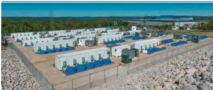
Figure 20 – Matrix flywheel system in Hazle Township, Pennsylvania. Source: Convergent Energy+ Power flywheels, photo credit: Eugene Hunt.
