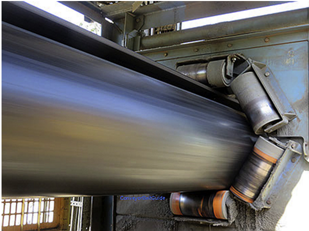
Fig. 4. Pipe conveyor (Image courtesy of Bridgestone Corporation).
