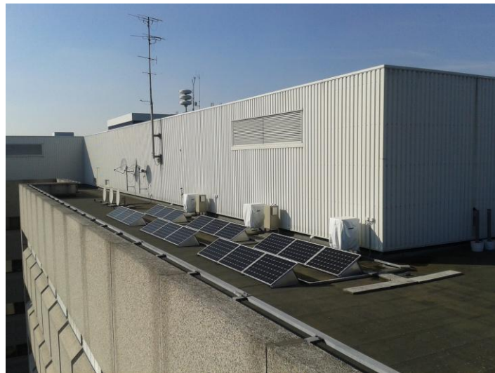
Figure 5. The experimental facility of SEAC.
