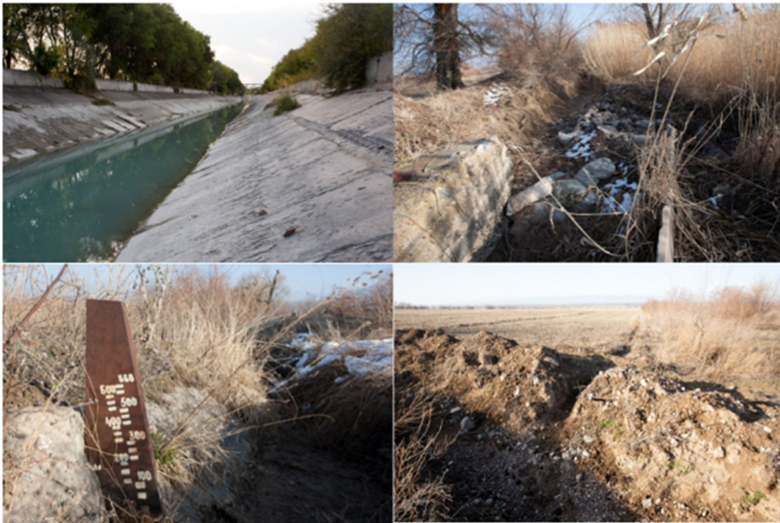
Fig. 3 Water system in Koram. Clockwise from top-left: (1) BAK, (2) MK Kuram, (3) water meter, (4) on-farm canal and irrigation ditch
