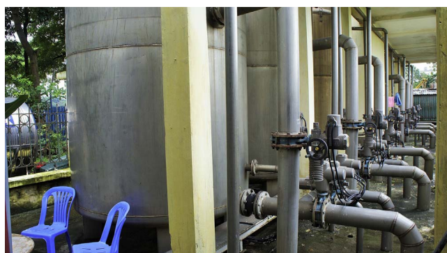
Fig. 5. HUD water supply plant in Linh Dam (authors).
