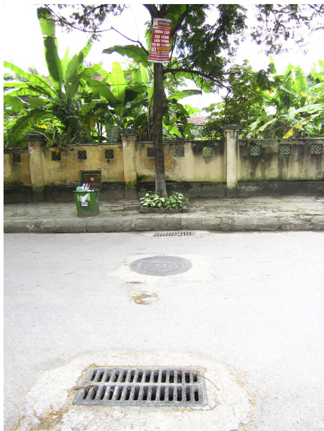
Fig. 4. Local sewerage system in My Dinh II (authors).
