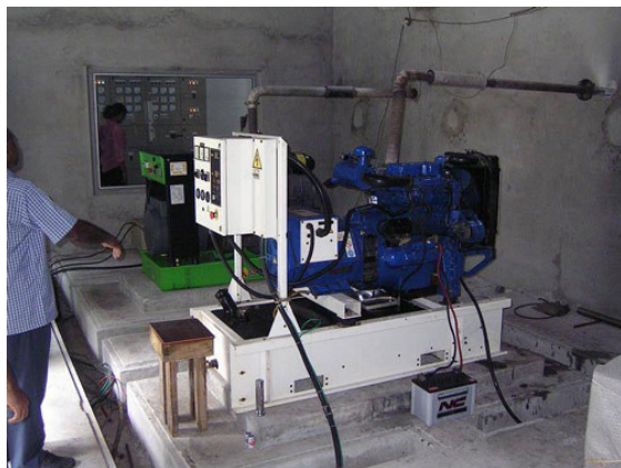
Figure 1: Existing diesel sets: back 31 kW, front 22 kW
