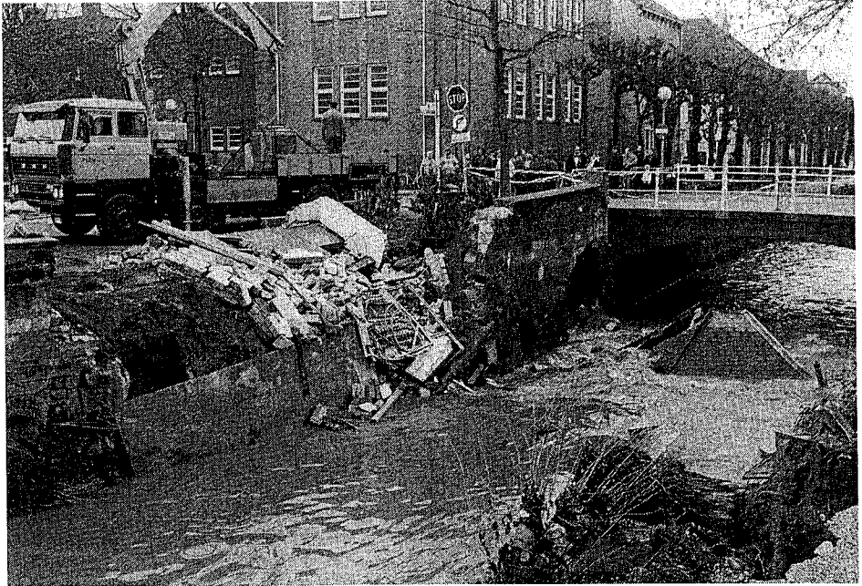
Photo 9.2 A few hours after the flood peak at the same location as on Photo 9.1: the electricity station and the sheet-pilings are devastated.
