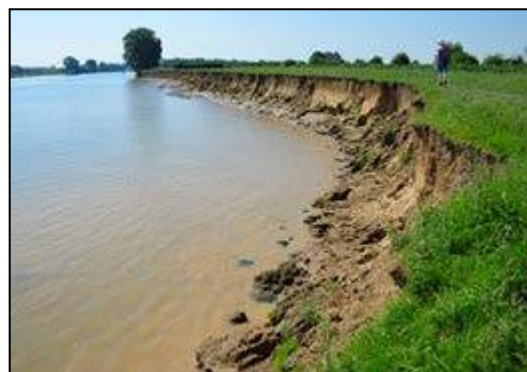
Figure 2. Bay-shaped erosion pattern characterized by high banks and contrasting erosion rates.
