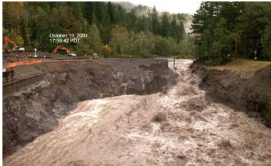
Figure 19. Controlled cofferdam failure at former Marmot Dam site on 19 October, 2007 (Major, 2012)
